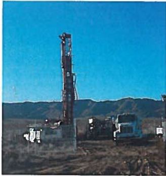
We access the aquifer by drilling wells, pumping water to storage tanks and delivering to your tap through pipelines in the street.
